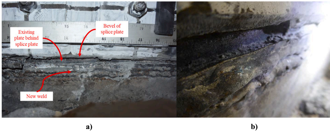
Fig. 15. Close-up picture of the fracture propagation at SWS from a) front view and b) side view.
